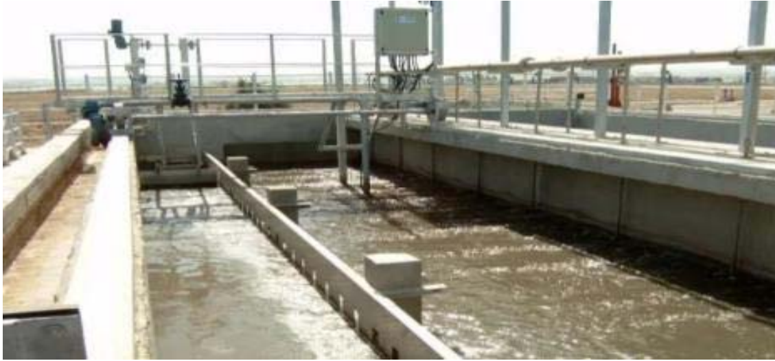
Figure 3-12: Typical View of Grit Chamber
