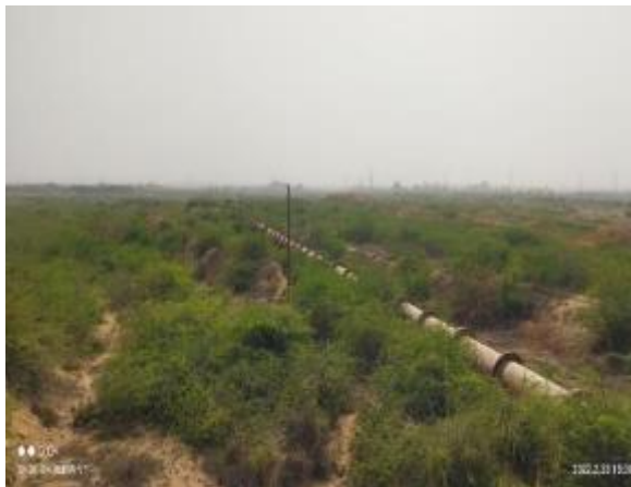
Dhabeji Rising Mains near Fore bay (High point)
