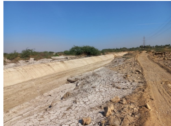
Scour pit at Downstream of GK Conduit in Creek-3
