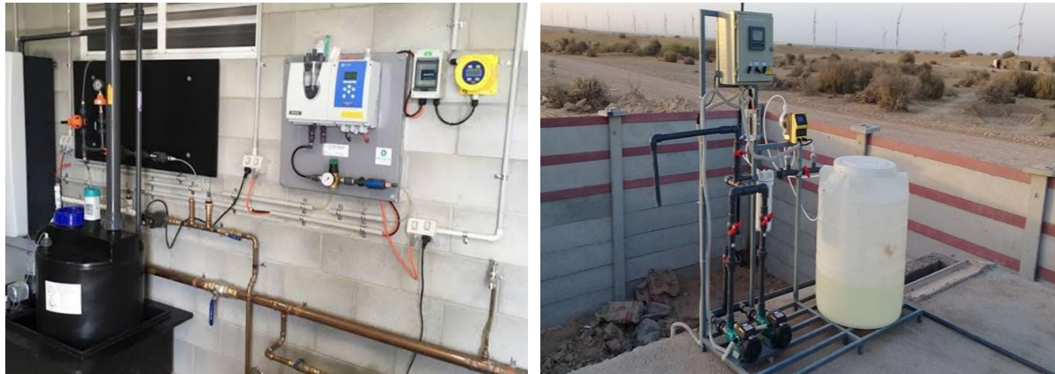
Figure A3-6: Typical Hypo-chlorinators to be Installed at Selected Pump Houses
